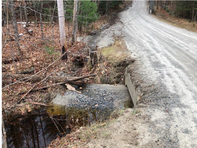
Significant sediment load conveyed to stream after road ditch failure, following large storm event in New London, NH. Fall, 2020.
