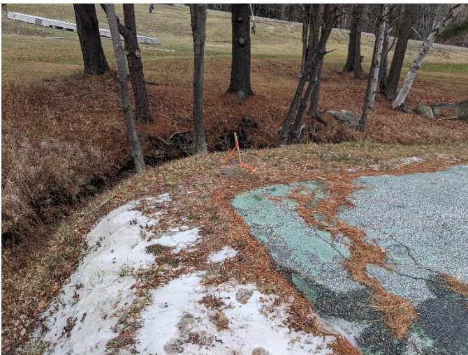
Entrenched 90-degree bend around parking lot embankment at Mount Sunapee Resort in Newbury, NH
