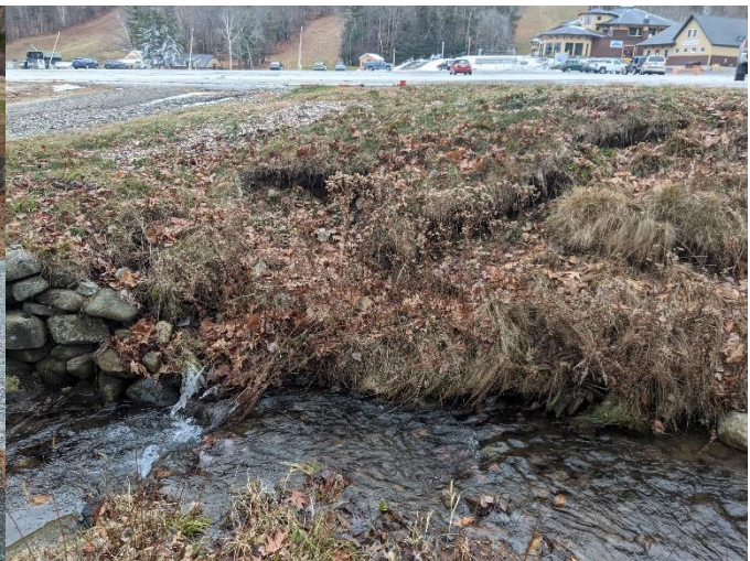
Erosion of parking lot embankment due to culvert flow contraction at Mount Sunapee Resort in Newbury, NH
