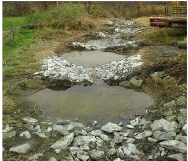
Photo of the step pool stormwater conveyance system, following construction and a rain event.
