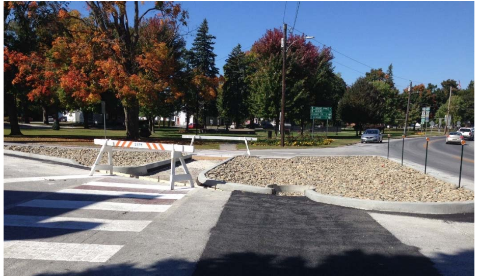
Construction of a stormwater infiltration area at the intersection of Academy St. and Route 7 in the Village of Swanton. This green infrastructure practice treats flow from 3/4-acre of road surface.
