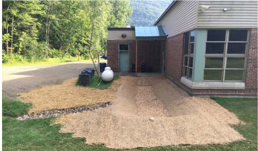
A bioretention area, shown above just after construction, captures and treats runoff from the school's rooftop.
