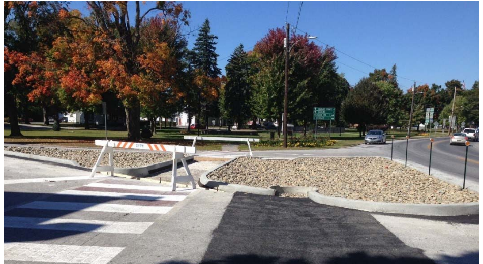
Construction of a stormwater infiltration area at the intersection of Academy St. and Route 7 in the Village of Swanton. This green infrastructure practice treats flow from 3/4-acre of road surface.
