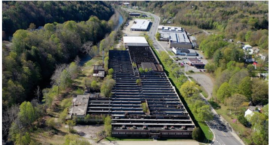
Drone photography of the Jones & Lamson property, with the Black River at left. Significant deterioration of the rooftop is visible.
