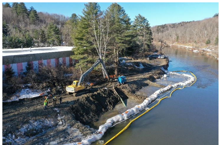
Top: Tar released to the ground surface on the bank of the Winooski River. Bottom: Excavation crews employ a coffer dam in the Winooski River while removing coal tar contaminated soils.
