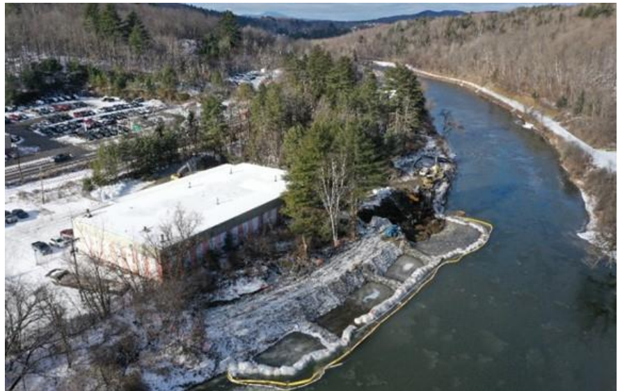
Copper dam and coal tar excavation cells along the Winooski River in Montpelier, Vermont. The former building supply retailer building has been redeveloped as the headquarters for a wastewater service contractor.
