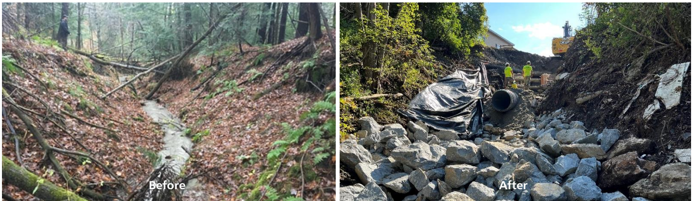
Left: The lower reach of the Deer Brook gully in November 2017. Gray water in the channel is due to fine sediment transport. Right: Construction of closed drainage system outlet improvements and energy-dissipating stone step pools in September 2022.
