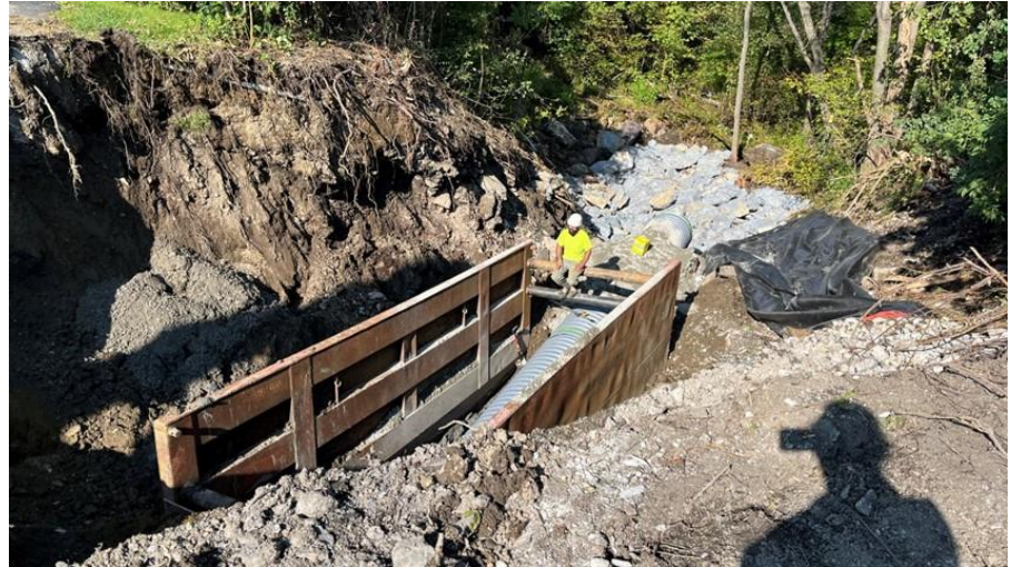
Installation of the new outfall and energy dissipating stone step pools in September 2022.
