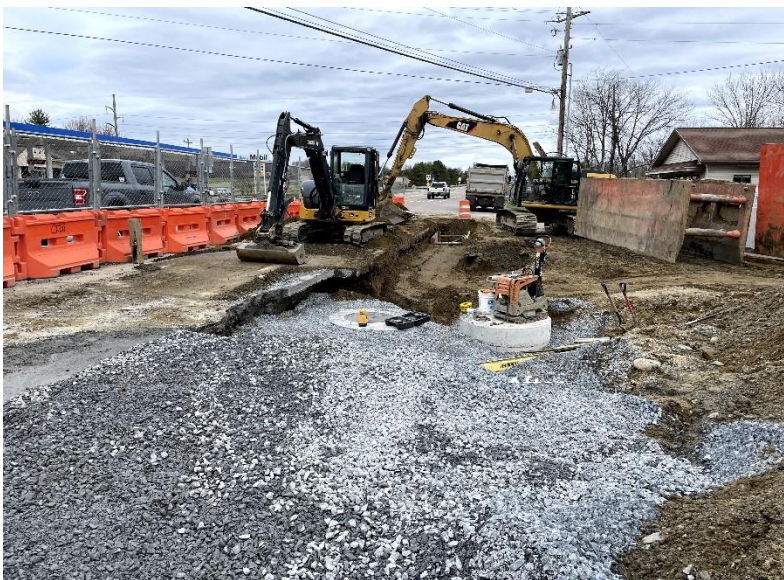
Installation of deep sump catch basin, drainage manhole, and associated stormwater culverts, April 2024
