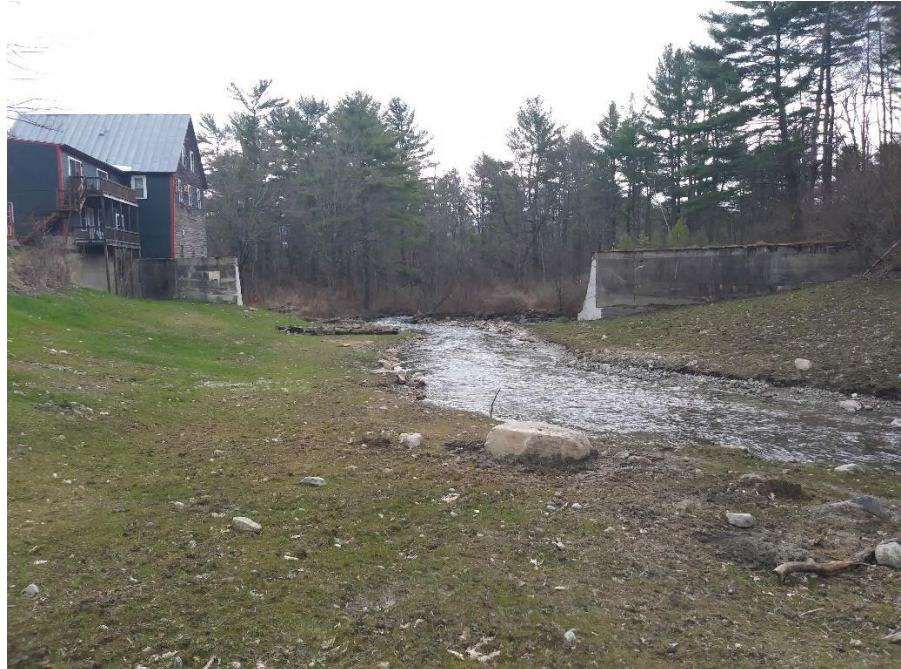
View of the project area, following the partial removal of the dam. The low-lying areas were seeded over with grass while the upland areas were planted with trees and shrubs.
