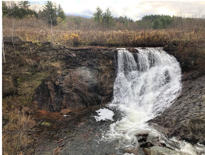
Looking upstream at the Johnsons Mill Dam along Bogue Branch in Bakersfield, Vermont in 2019.
