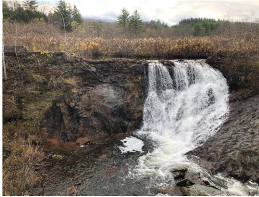
Looking upstream at the Johnsons Mill Dam along Bogue Branch in Bakersfield, Vermont in 2019.
