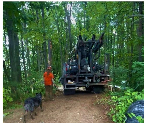
Drill rig transportation through a wetland with temporary road construction at the Commerce Street Superfund Site in Williston, Vermont.
