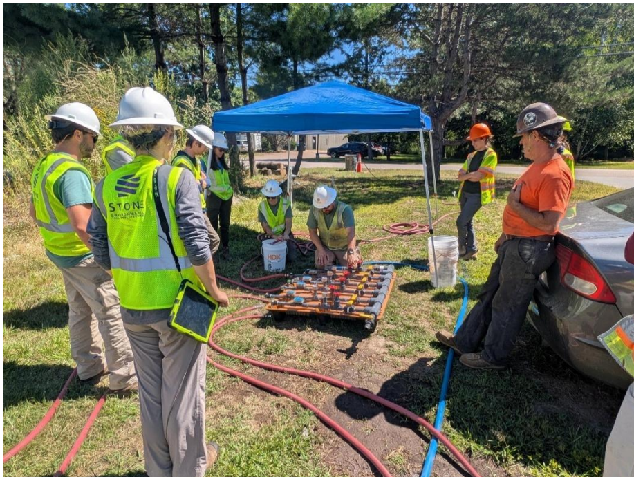
Stone, Platform, and VT DEC staff members review injection procedures at one manifolded location on the Commerce Street Superfund Site in Williston, Vermont.
