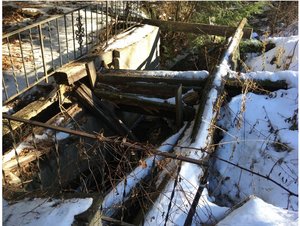
The project area, showing partially collapsed wood and metal construction.
