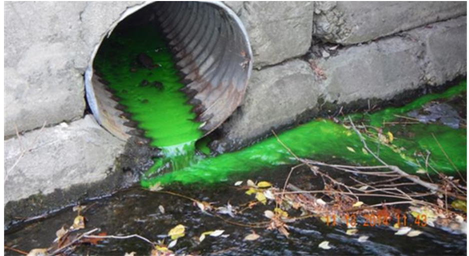
Dye flushed down a toilet in Barton, Vermont discharges to a stream, confirming a sanitary wastewater connection. Direct sanitary connections from two houses to the storm drain were eliminated.
