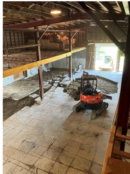
Site work during the implementation of the CAP and SICP. Contractors work to remove a portion of the existing floor.
