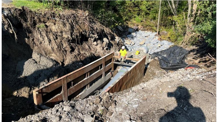
Installation of the new outfall and energy dissipating stone step pools on September 14, 2022.
