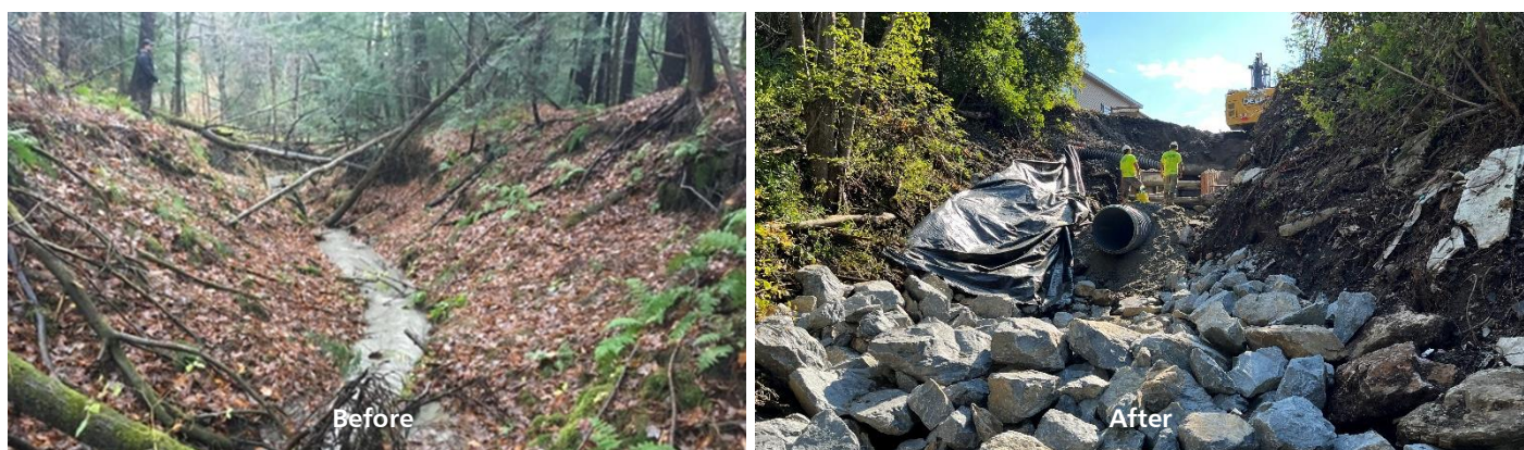
Left: Existing condition in the lower reach of Deer Brook gully, seen in November 2017. Gray-colored water in the channel is due to fine sediment transport during a moderate rain event. Right: Construction of new outfall and energy-dissipating stone step pools in September 2022.
