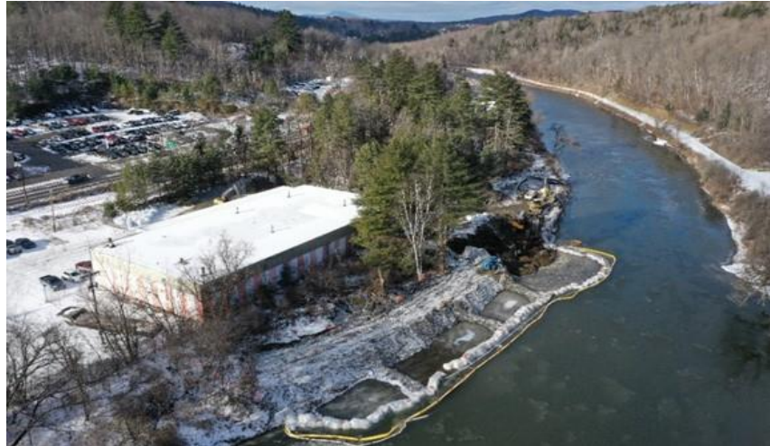
Coffer dam and coal tar excavation cells along the bank of the Winooski River in Montpelier, Vermont. The former building supply retailer building has been redeveloped as the headquarters for a wastewater service contractor.
