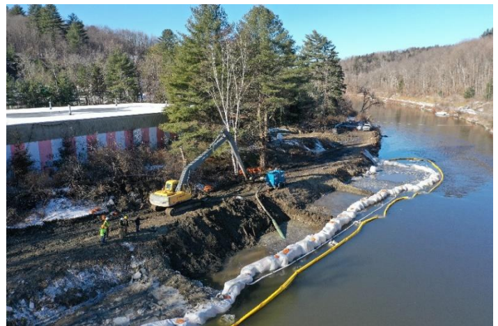
Top: Tar released to the ground surface on the bank of the Winooski River. Bottom: Excavation crews employ a coffer dam in the Winooski River while removing coal tar contaminated soils. Photos by Stone Environmental
