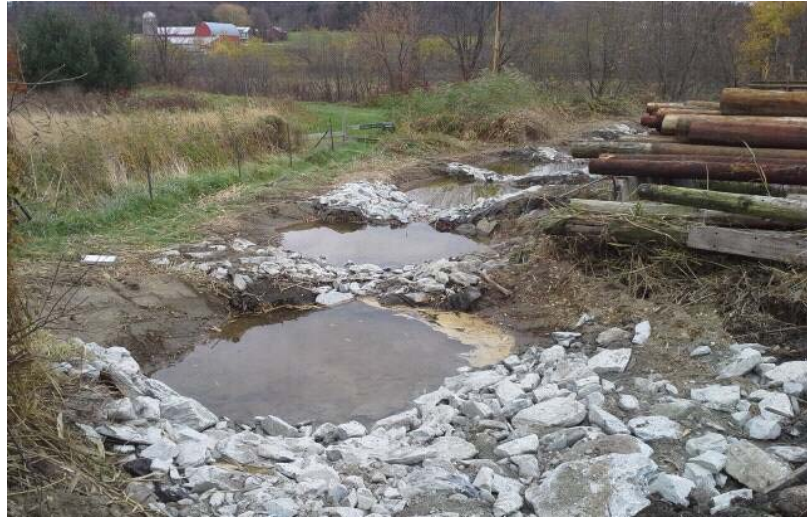
Photo of the step pool stormwater conveyance system, following construction and a rain event.
